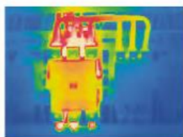
Power Distribution cabinet inspection
