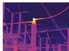
Connector overheating inspection
